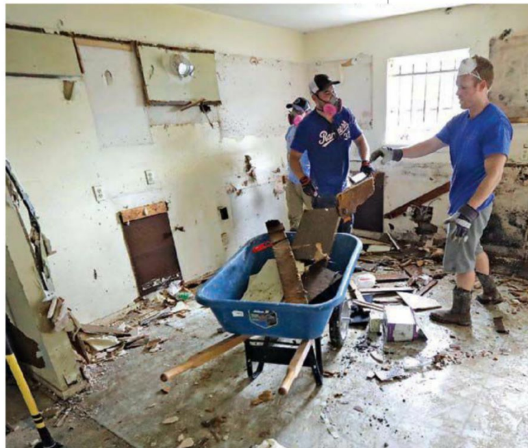
▼ A cleanup crew deals with the aftermath of Harvey in Houston
